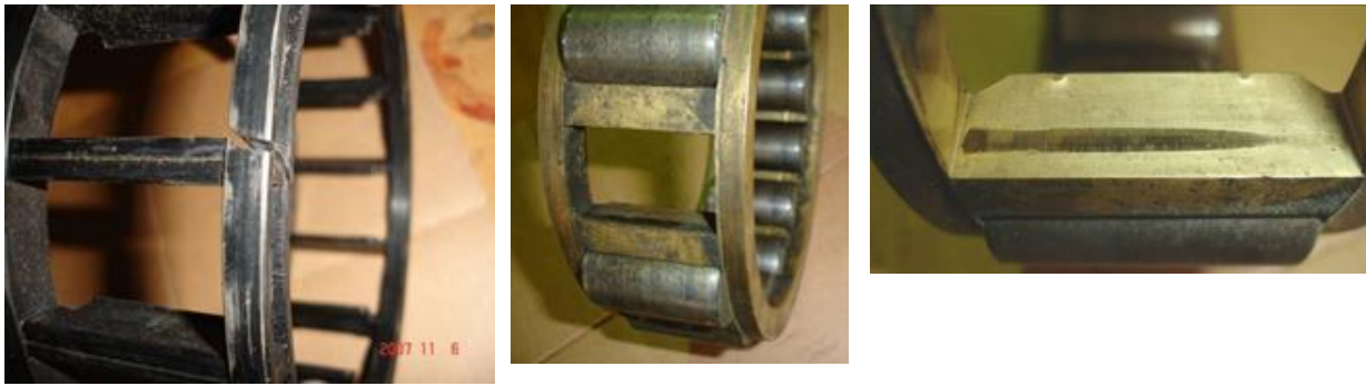
Fig. 2.11. Destruction and wear of cage rings and bridge sections
